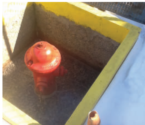
An old-style industrial hydrant with only two 2½-inch connections. This hydrant for some reason was installed in the ground and is difficult to use.
