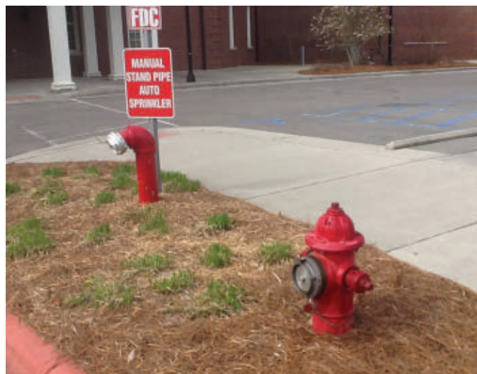
A hydrant well located next to a fire department connection, but how much flow can we take from it? (Photos by author.)
