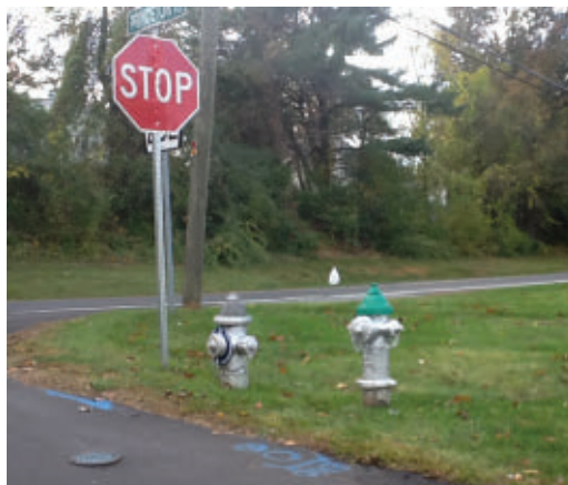
Two adjoining hydrants on two separate systems. What flows are available from which one?
